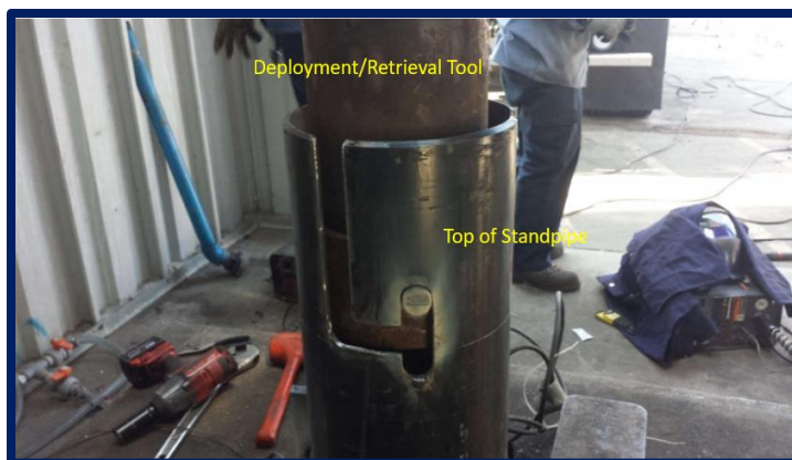
Figure 1: Standpipe with "L" Slot and Deployment/Retrieval tool (with pin slid into L-slot) deploying free-standing, dual-packer, well modification system into City Yard Well in 2016.
